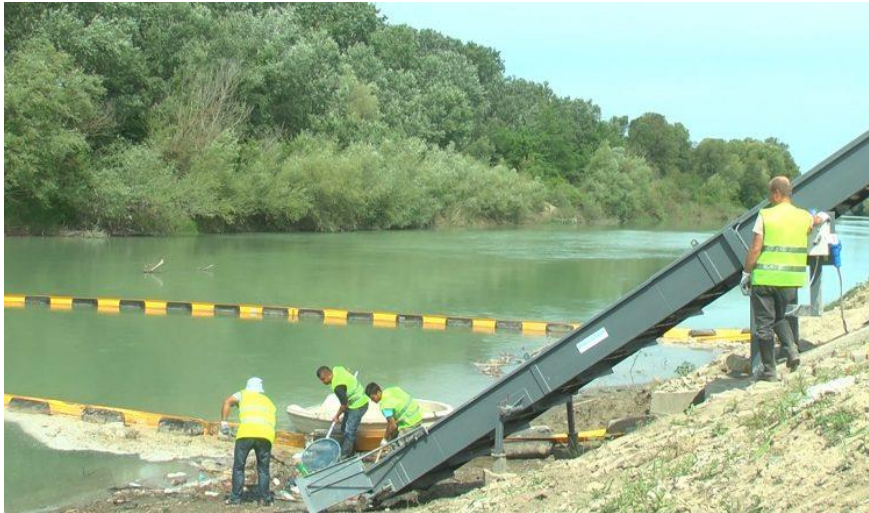
Figure 12: Photo from the machinery installed for the collection of waste in Shkumbini River
